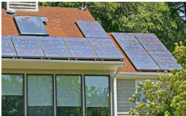
Photovoltaic Roof Top Solar Panel System
