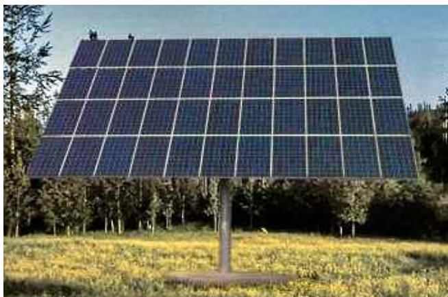
Photovoltaic Pole Mounted Tracker Solar System (Ground)
