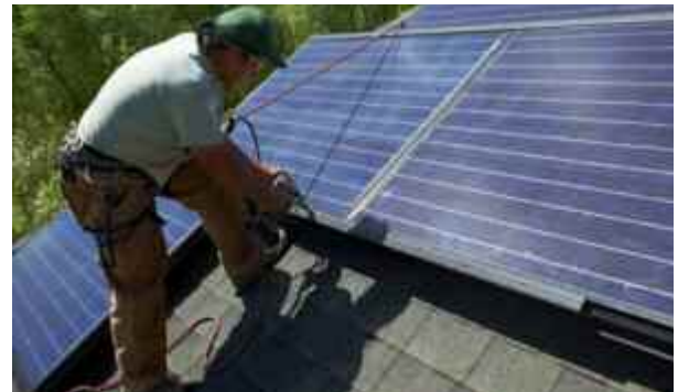
Commercial application of a complete Solar Energy System - Solar PV Roof Top Panels
